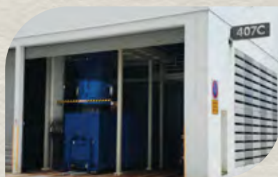
Pneumatic Waste Conveyance System (PWCS)
