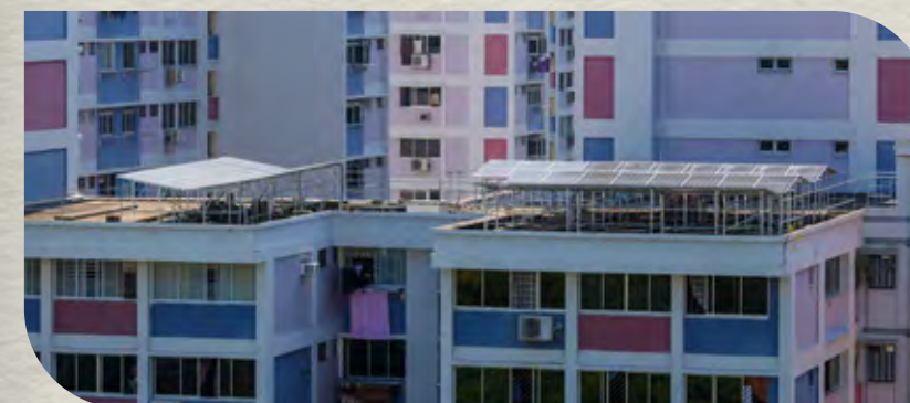
Solar panels installed in HDB estates
